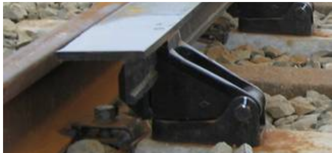
Anti-derailing Guard Rail
